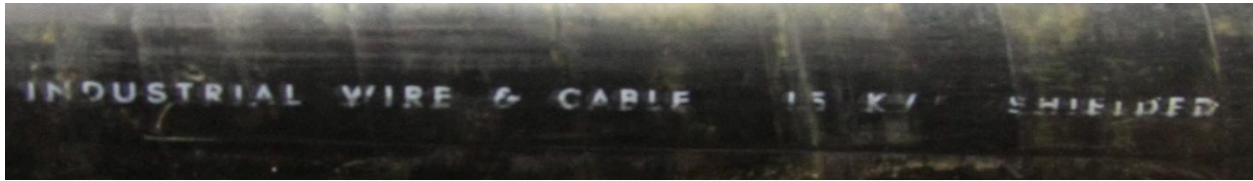
Figure 3: Manufacturer Identification Found under the Tape Neutral
