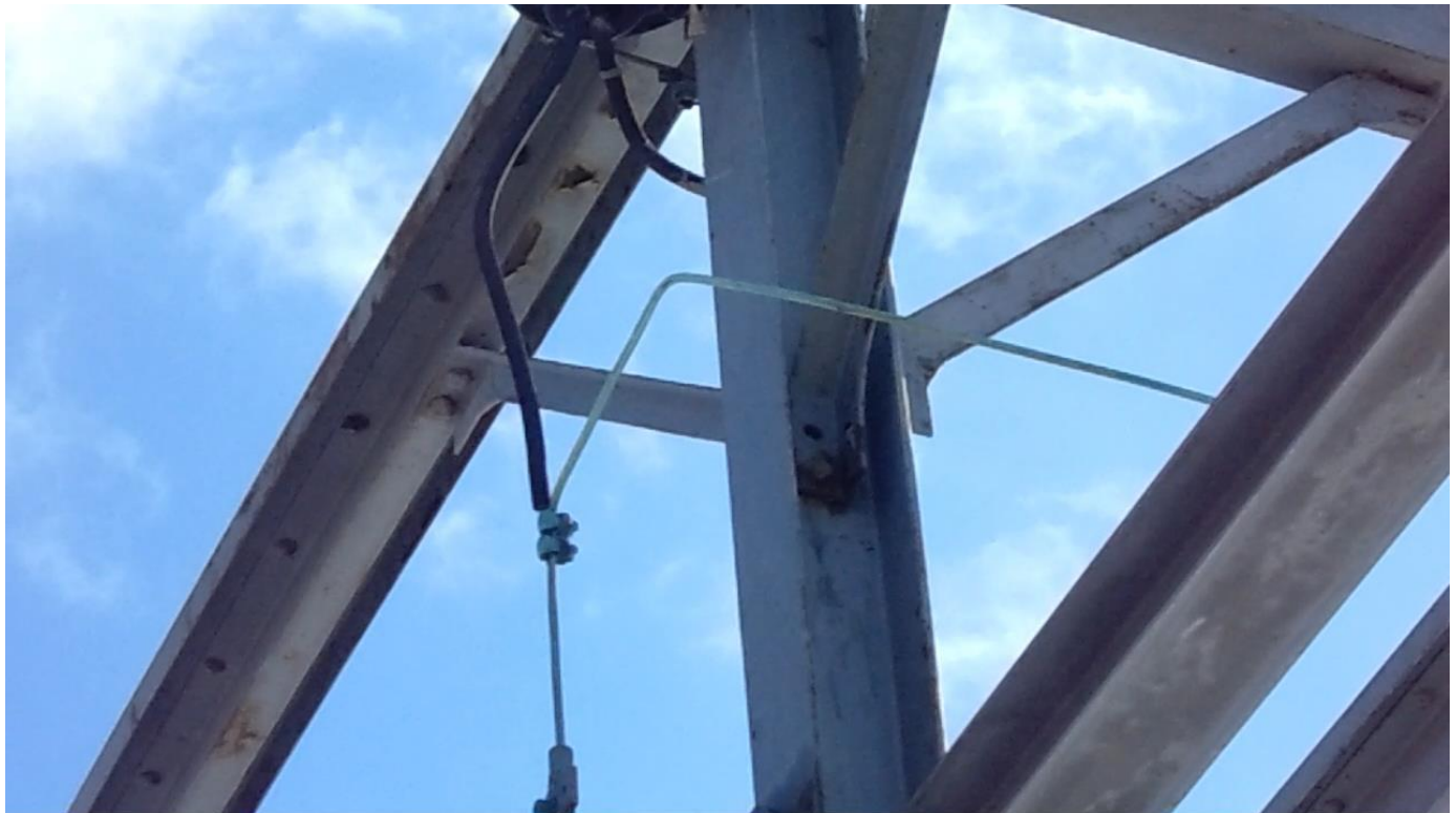
Photograph 6 – Missing Connection Bolt
