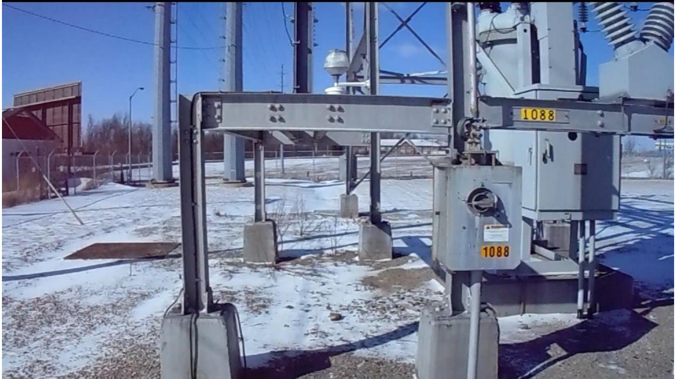
Photograph 8 – Heaved Concrete Pier
