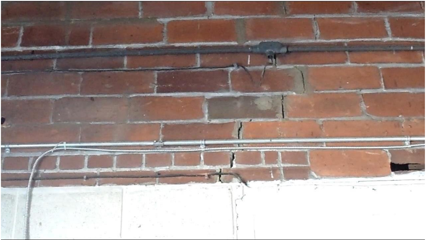
Photograph 3 – Control Building Wall Cracks
