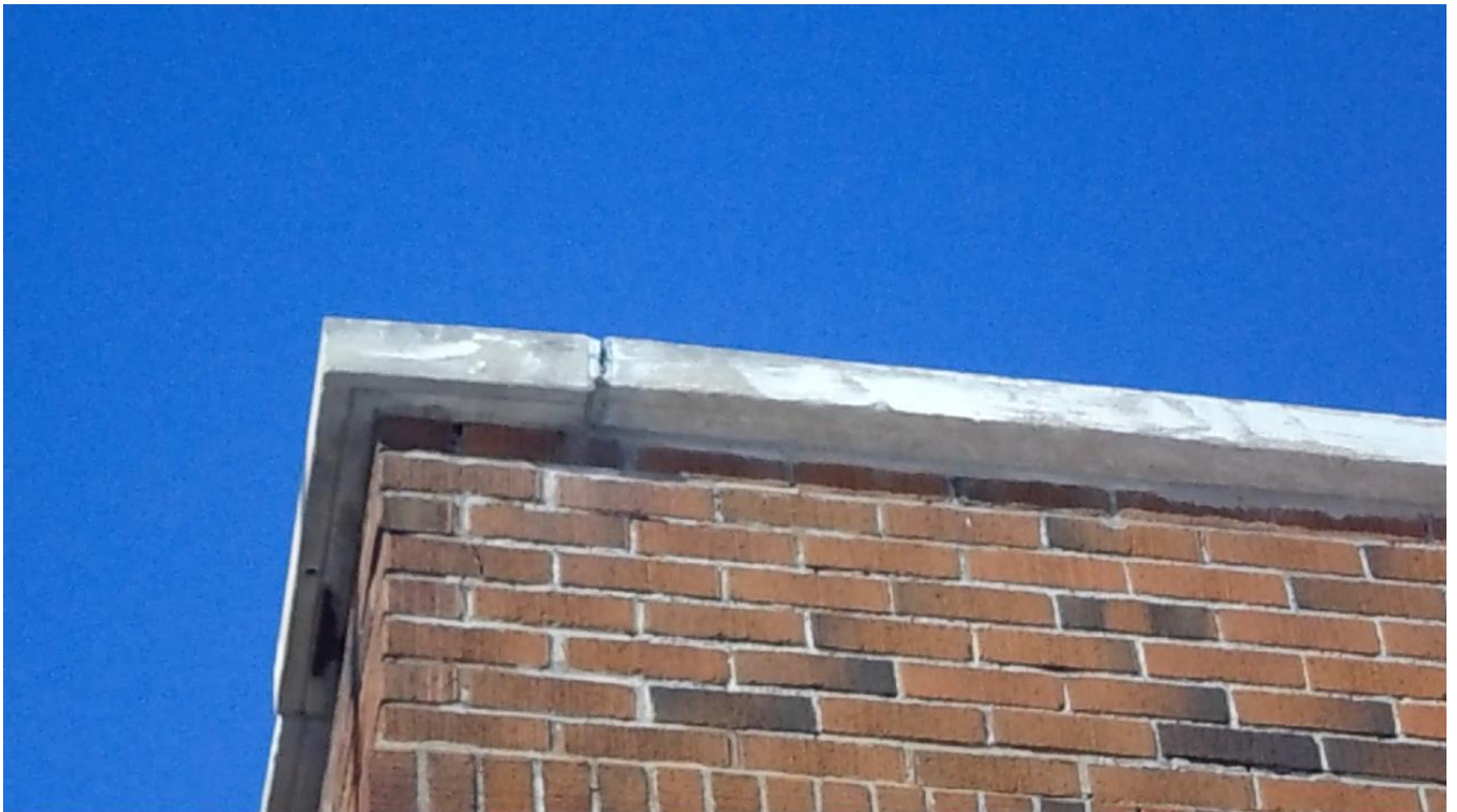
Photograph 4 – Control Building Parapet Joint Failure
