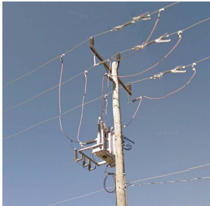
Figure 5.4.6.x-1 SCADA Controlled Recloser Installation
