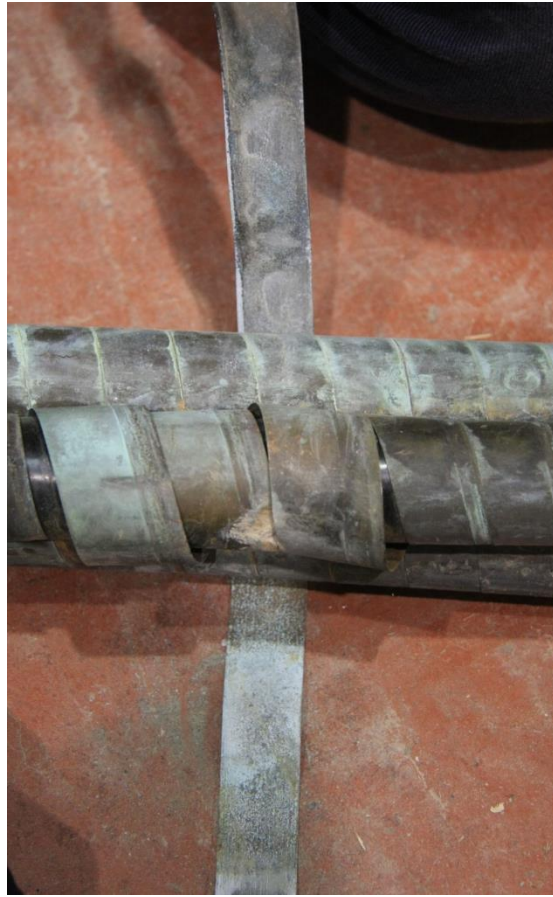
Figure 14: Only Minor Damage Found under the Tie
